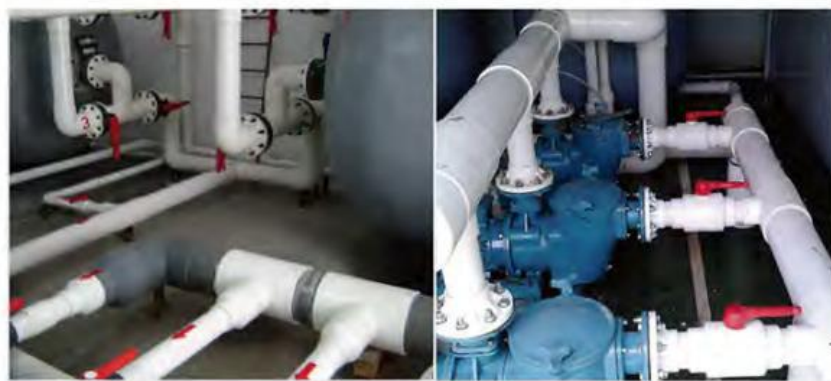
Standard water treatment room ensures safe and clean water quality of disassembled swimming pool
